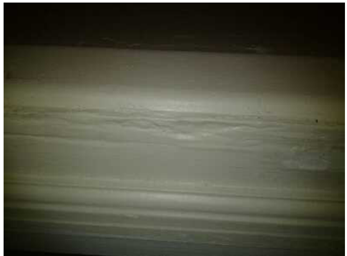
termite damage in bath door jamb
