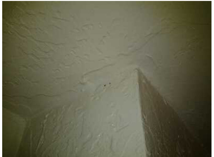
termite pinholes ceiling in kitchen
