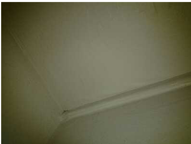
water damage ceiling of front bedroom closet
