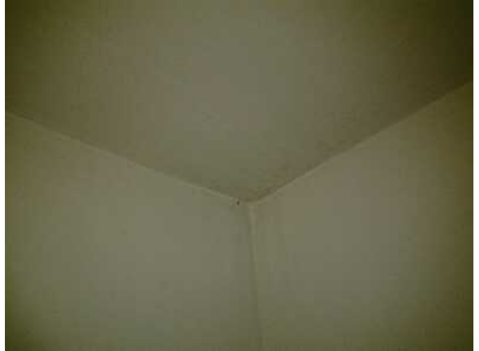
termite pinholes northeast corner ceiling of bath
