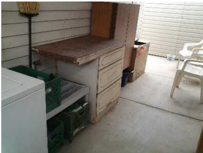
patio walls obstructed and water slopes towards house
