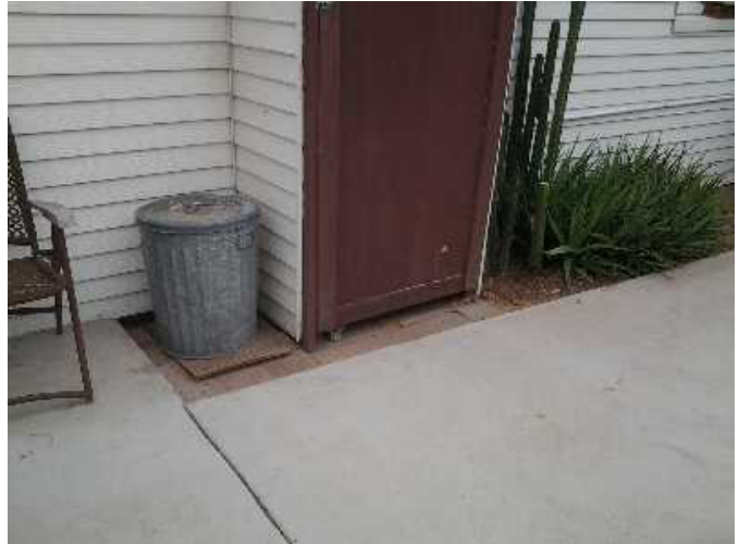
water slopes towards house
