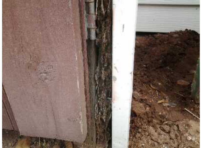
termite damage on water heater shed
