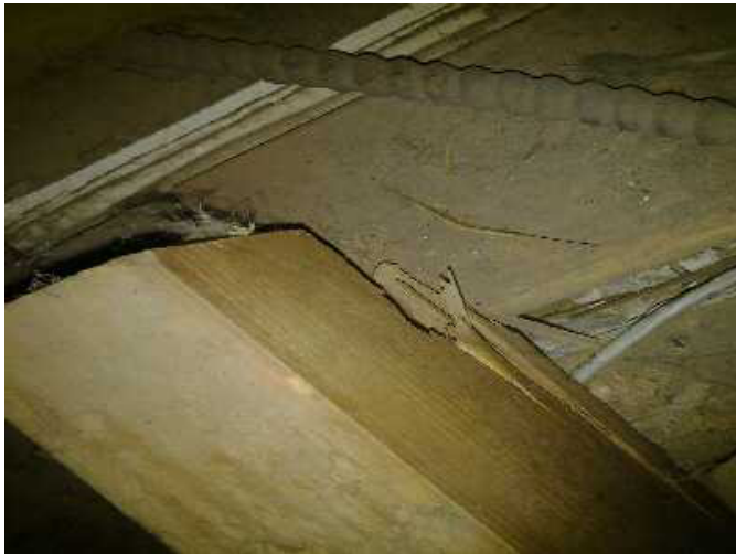
termite damage in attic
