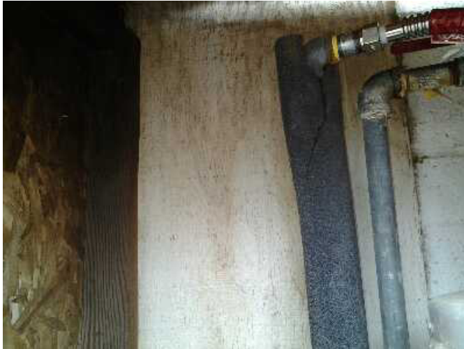
water stains water heater shed
