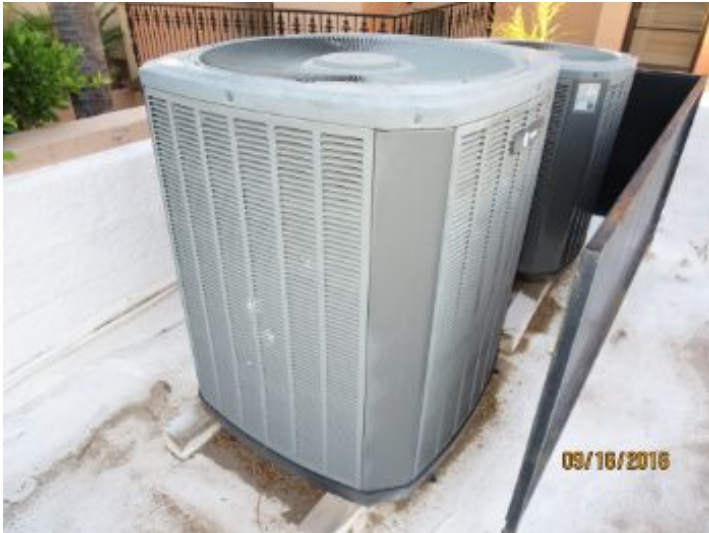
Provided cold air at time of inspection
