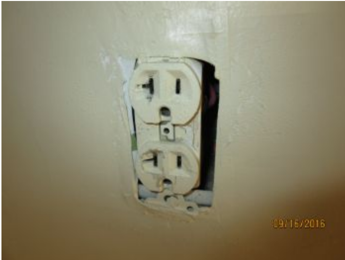
Outlet cover missing
