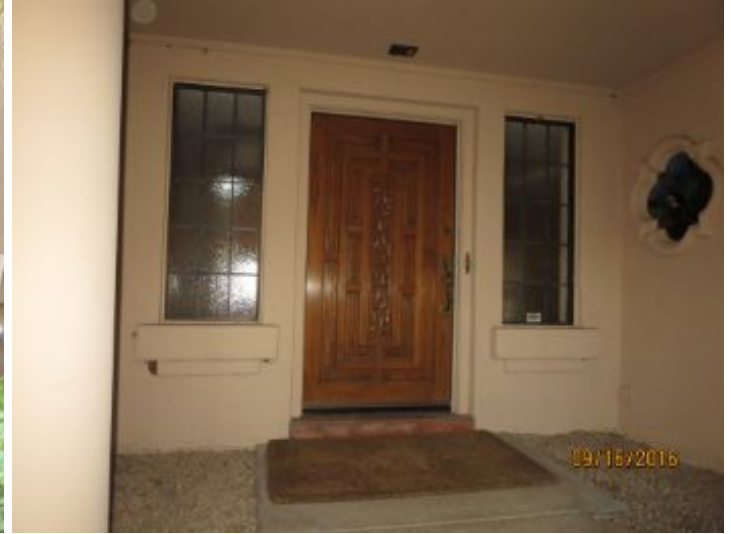
Front entryway appeared to be in good condition at time of inspection.
