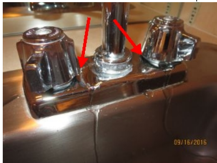
Both hot and cold faucets leak at stem seal
