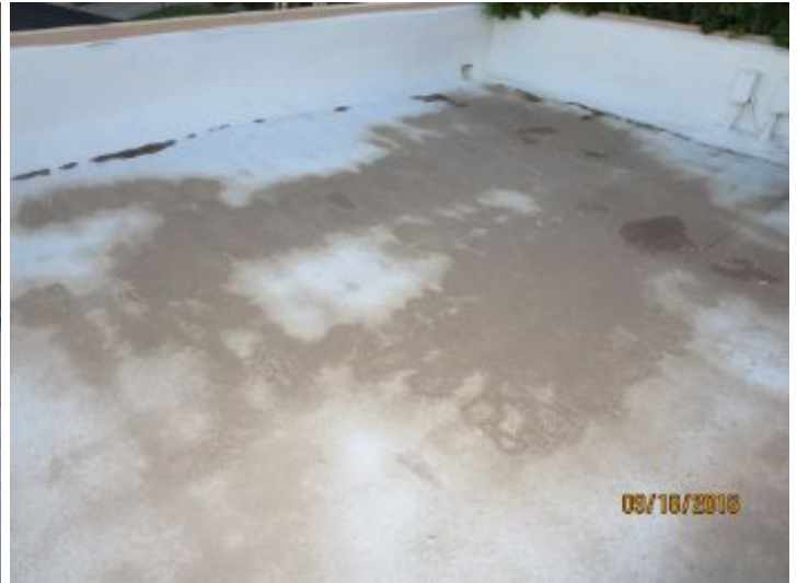
Ponding noted in one or more location(s)
