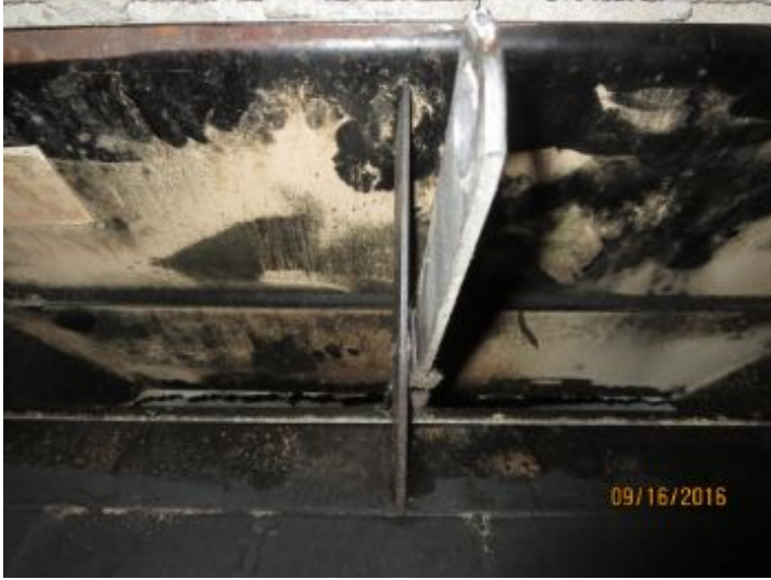
Damper was operational at time of inspection.
