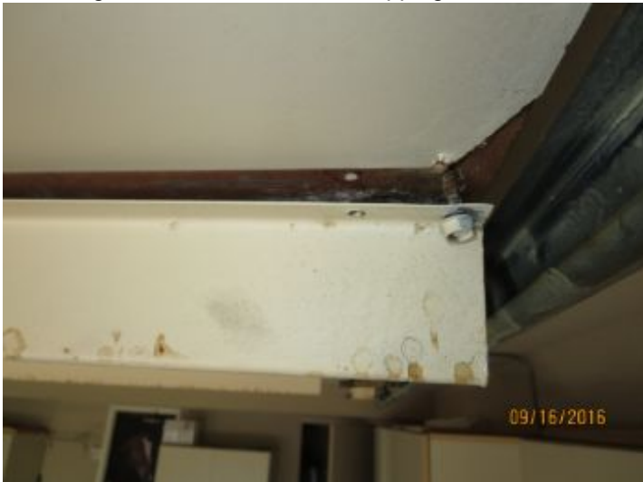
Loose garage door components noted
