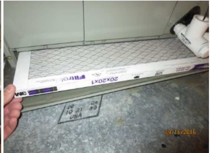
Furnace filter location: Furnace base. Size: 20" x 20"
