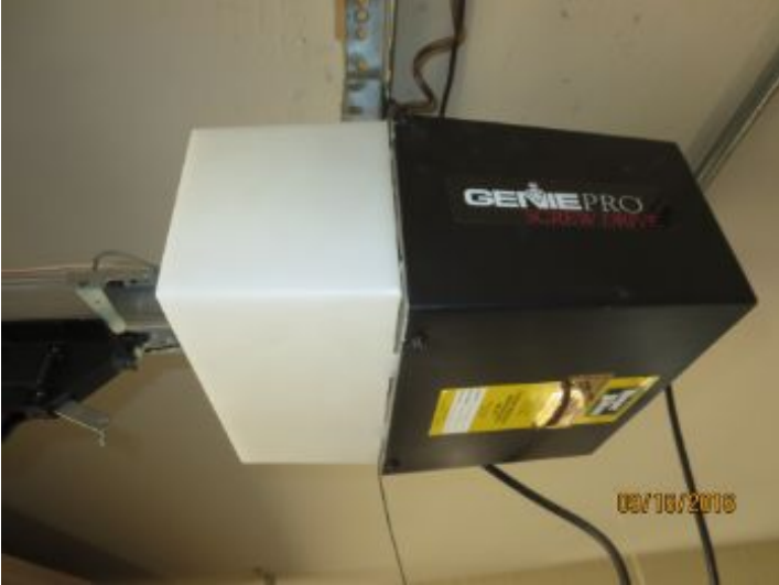
Garage door opener operated at time of inspection.
