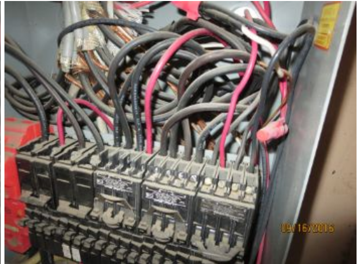
The branch wires visible in the panel are copper and are in satisfactory condition.
