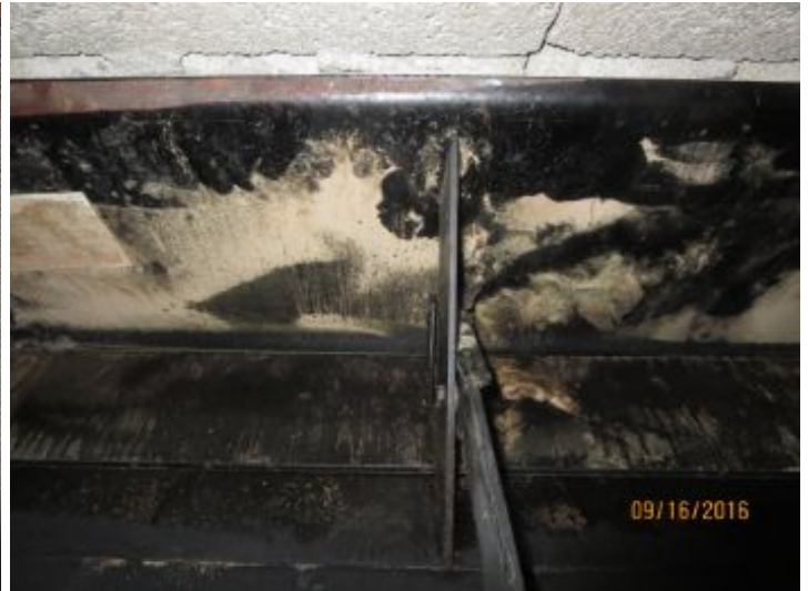
Damper was operational at time of inspection.
