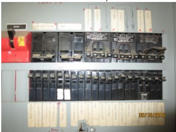
Breakers appear to be marked/identified.
