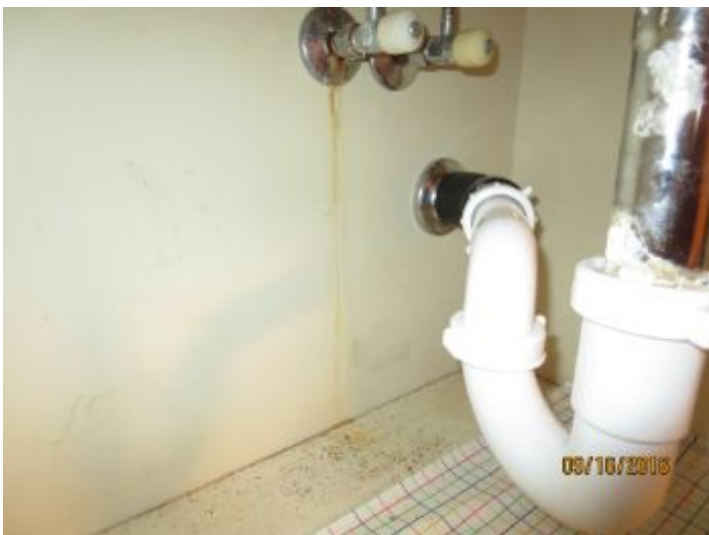
Evidence of past leaking noted at plumbing connection.
