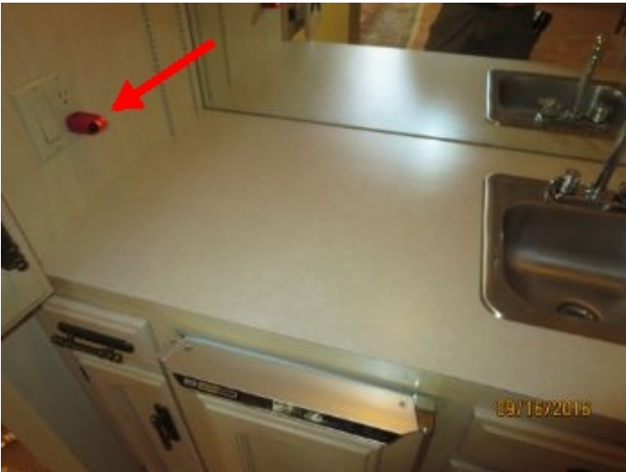
Recommend GFCI at outlet next to wet bar sink.
