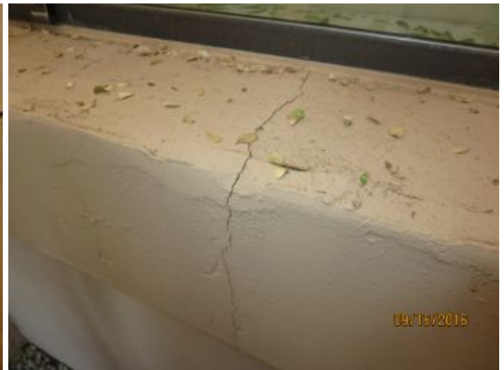
Common cracking noted
