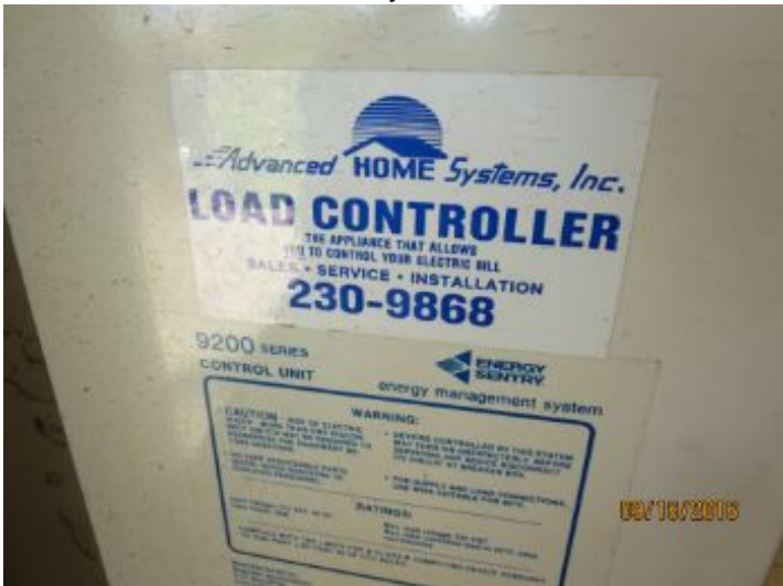
"Load Control Center" installed on interior garage wall. Not part of home inspection - recommend further review by a qualified electrician.
