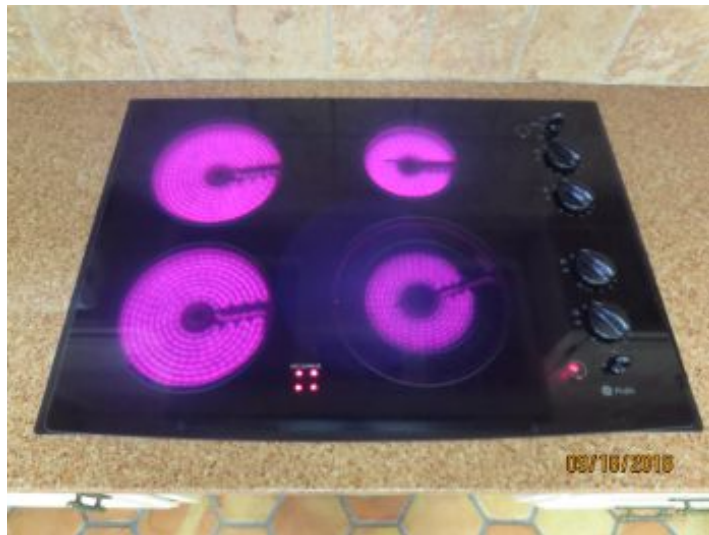
All 4 burners heated up when switched to the on position at time of inspection.
