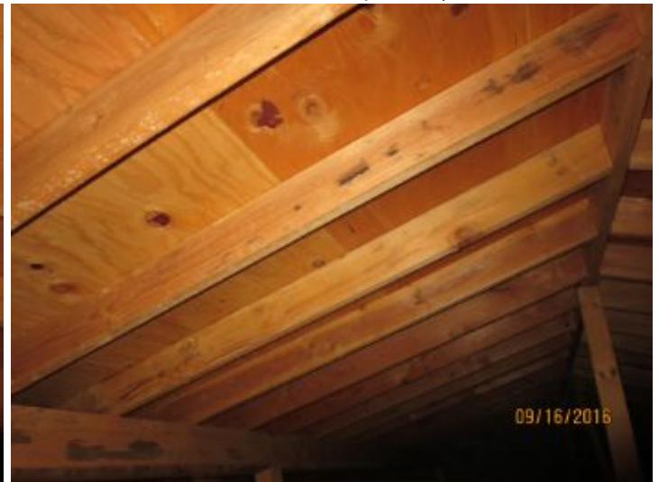
Roof structure appeared to be in good condition with no visible evidence of water stains or structural issues in the areas that I had access to.
