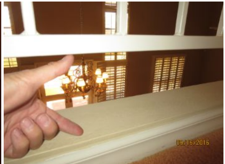
Current building standards allow a maximum of 4 inches between spindle spacing and below railings. This may not have been the standard when this home was built. Possible safety hazard to small children falling through openings and/or getting their heads stuck between spindles. Recommend upgrades to enhance safety of occupants and guests.
