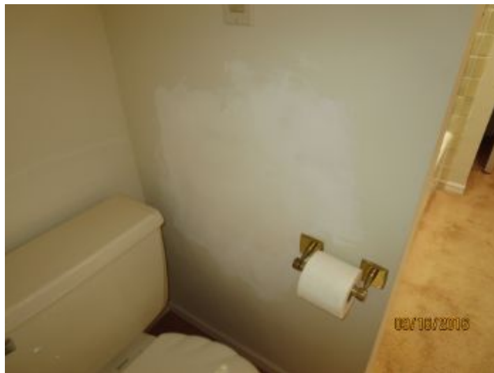
Patched areas noted
