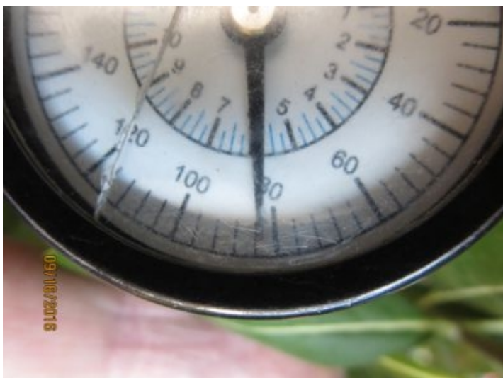
Water pressure was a bit high at 83 PSI. Recommend adjusting pressure regulator down to bring water pressure down into the mid 70 PSI range.
