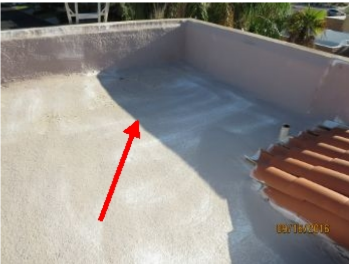
Scupper in northeast corner of upper roof has been sealed with concrete. It appears that water pools in this area when it rains. Recommend review by roofing contractor.
