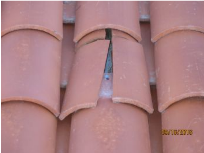
Broken tiles noted
