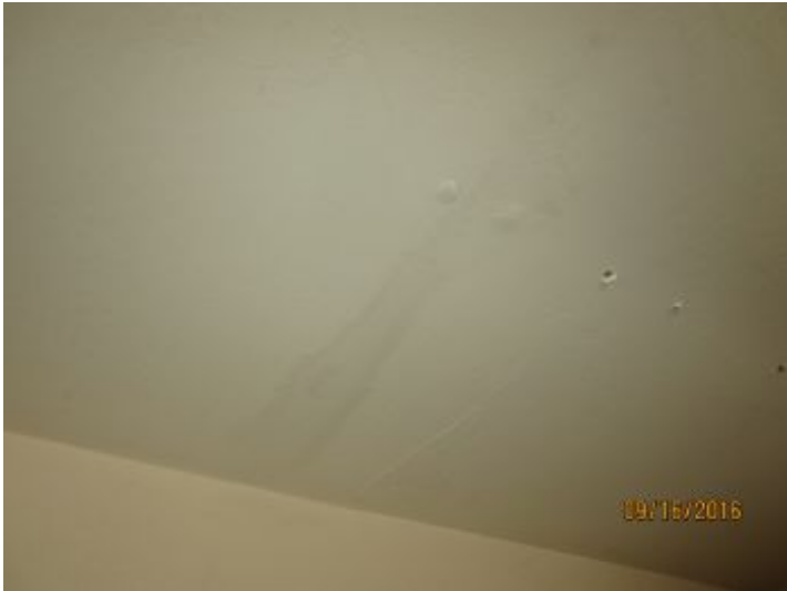
Water damage noted at garage ceiling, did not verify if leak is active or has been repaired, review and repairs are recommended by a qualified roofing contractor.
