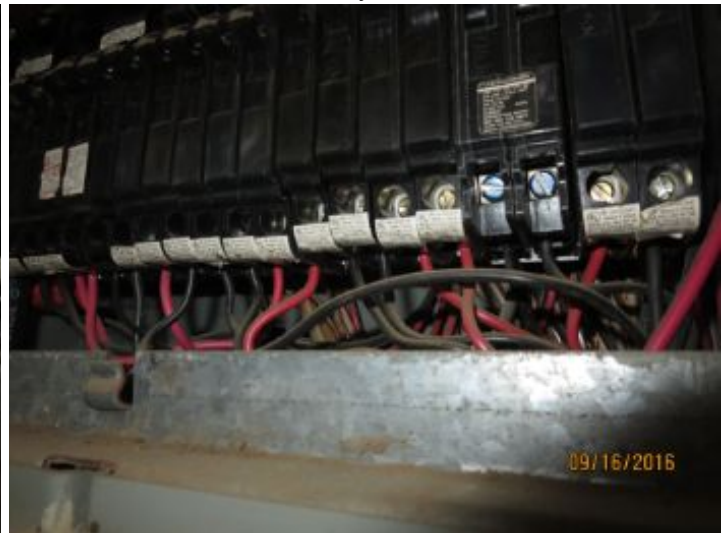
The branch wires visible in the panel are copper and are in satisfactory condition.
