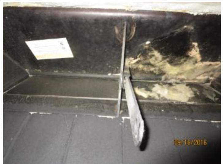
Damper operated at the time of inspection
