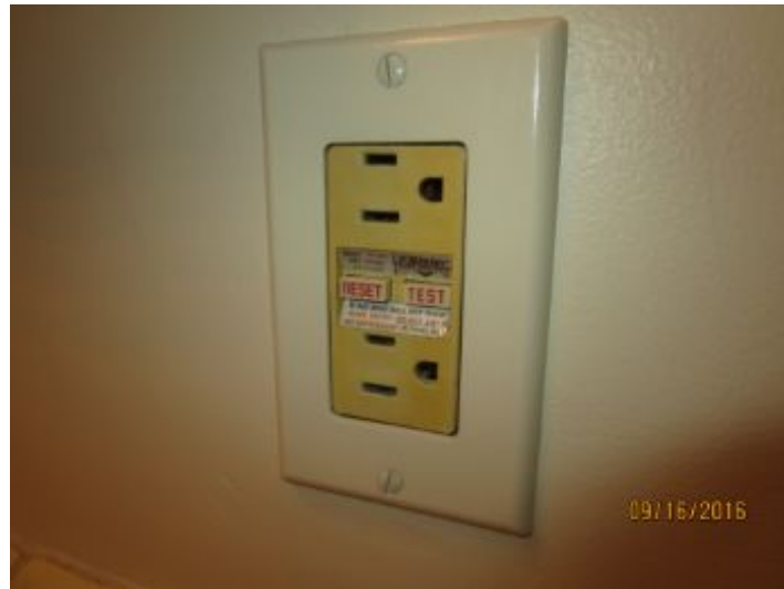
GFCI reset for exterior outlets appears to be located on back wall of garage
