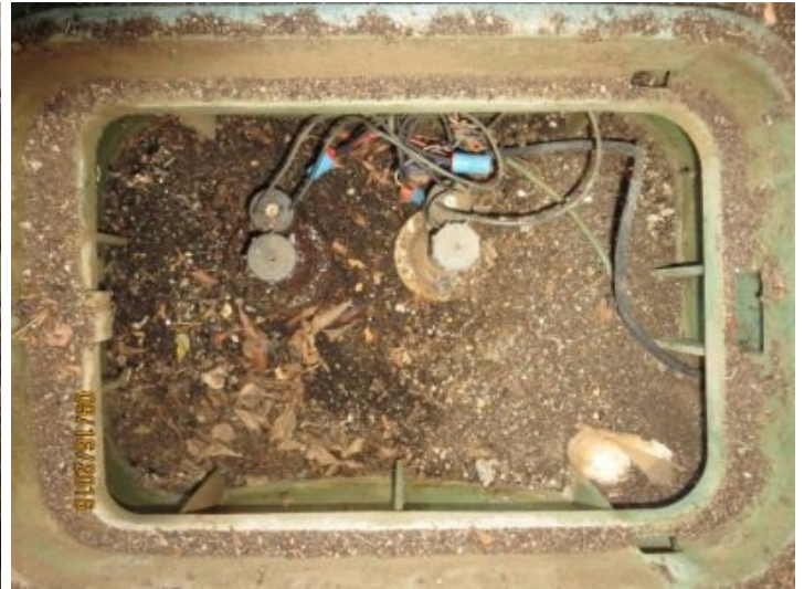
Valve box 1 location: East side of garage
