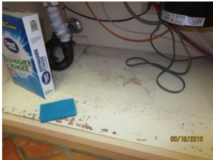
Evidence of past leaking under kitchen sink
