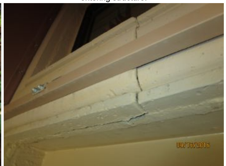
Common cracking noted
