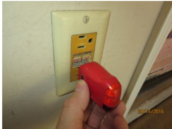
GFCI outlet by interior garage door did not trip when tested. This also appears to be the GFCI reset location for the exterior outlets which did not trip when tested. Suggest review/repair by qualified electrician.
