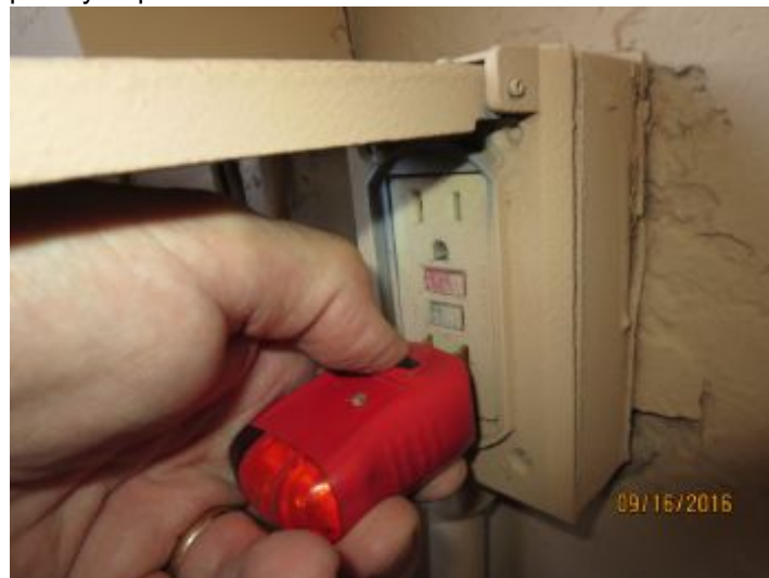
Exterior GFCI outlets did not trip when tested. The exterior electrical outlets appear to be controlled by the non-functioning GFCI outlet on the back wall of the garage. Recommend further review/repair by a qualified electrician.
