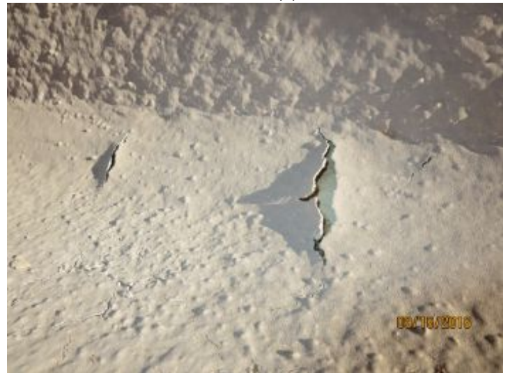
Holes/deterioration noted in foam in one or more location(s) Recommend further review/repair by a qualified roofing contractor.
