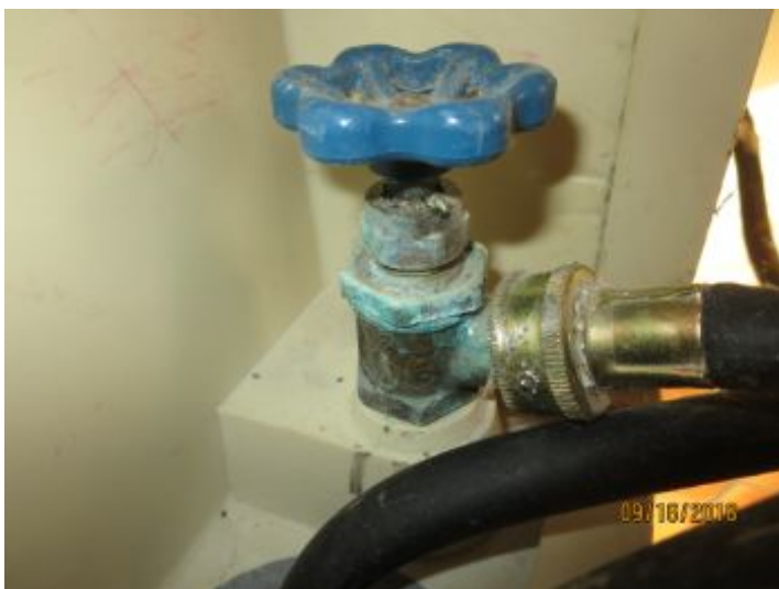
Recommend upgrading the hot and cold water shutoff gate valves to more reliable ball valves. Gate valves that are not used on a regular basis tend to build up mineral deposits which can, over time, prevent the valve from completely stopping the water flow when the valve is turned off.
