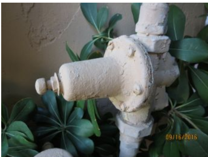
Water pressure was a bit high at 83 PSI. Recommend adjusting pressure regulator down to bring water pressure down into the mid 70 PSI range.
