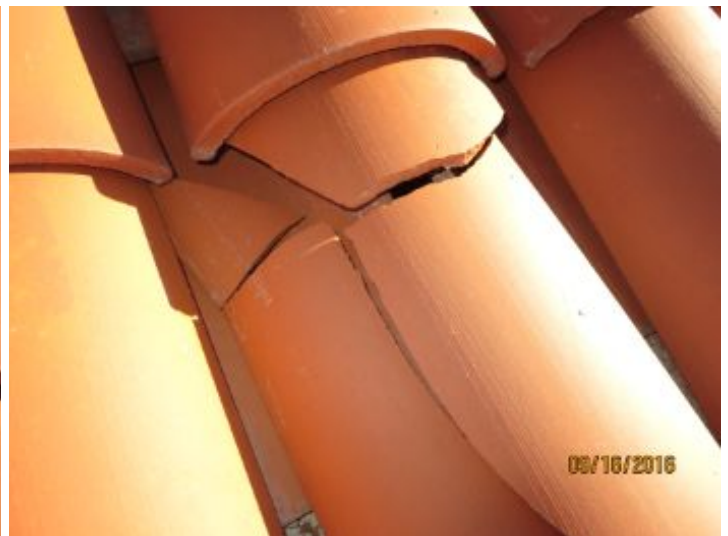
Broken tiles noted
