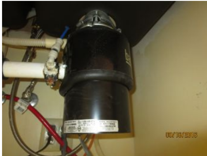
Disposal operated at time of inspection.
