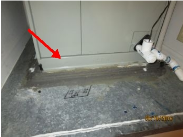
Furnace filter location: Furnace base. Size: 20" x 20"
