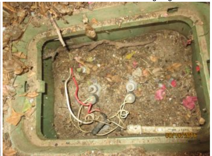
Valve box 2 location: Southeast corner of back patio
