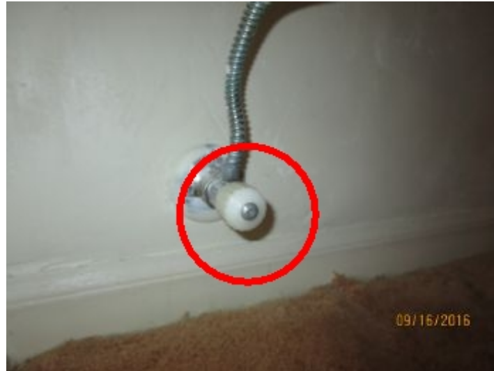
Water shutoffs for toilets located on left side of toilets
