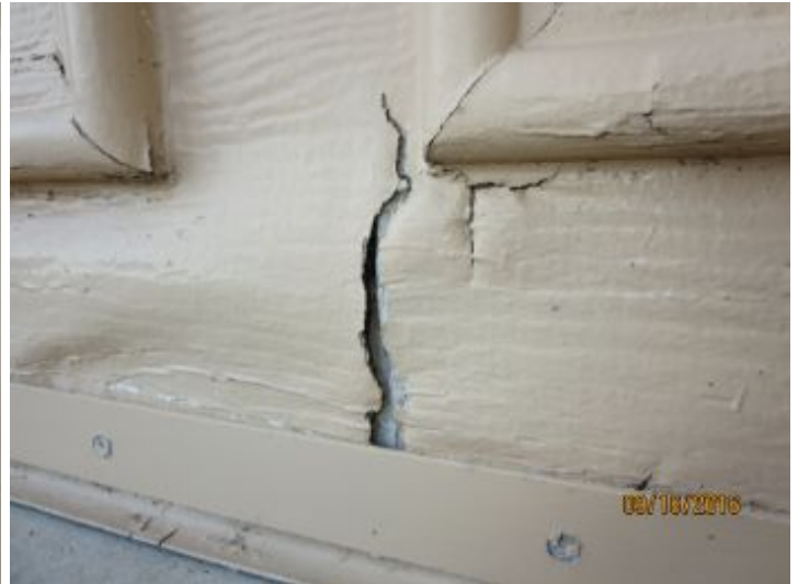
Damaged/deteriorated exterior garage door panels noted.
