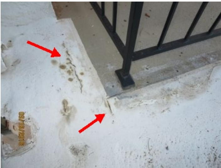
Cracking noted in foam around railings on lower roof
