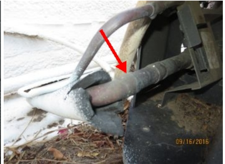
Deteriorated/missing insulation in areas. Recommend replacing the pipe wrap insulation to enhance efficiency of A/C system
