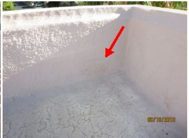
Scupper in northeast corner of upper roof has been sealed with concrete. It appears that water pools in this area when it rains. Recommend review by roofing contractor.
