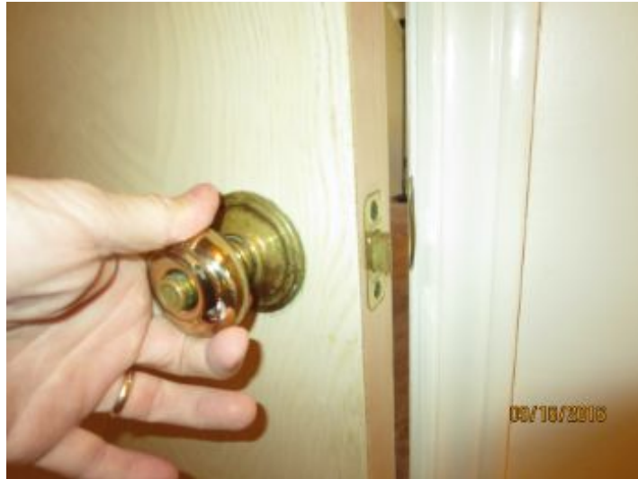
Guest bath door did not latch in 2nd floor northeast guest bath - striker plate needs adjustment
