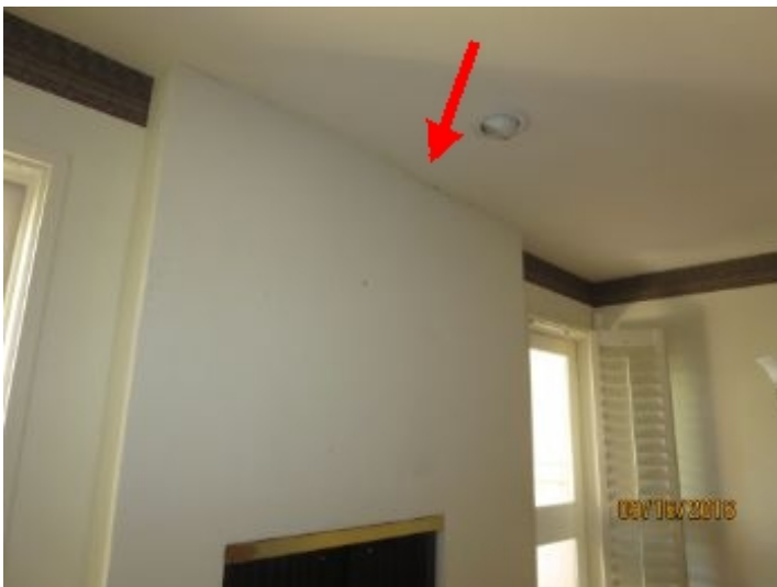
Evidence of past leaking at ceiling above fireplace in northeast bedroom.,did not confirm that leak has been properly repaired. Recommend monitor area after heavy rain and repair as needed by qualified roofing contractors.
