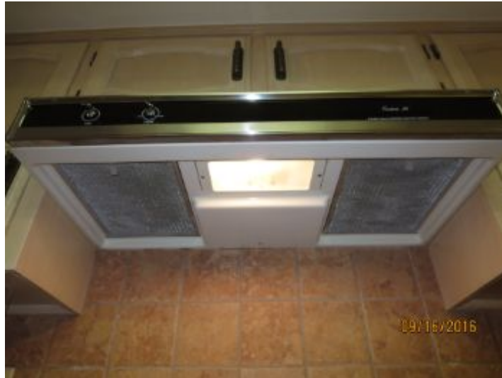
Exhaust fan and work light operated at time of inspection
