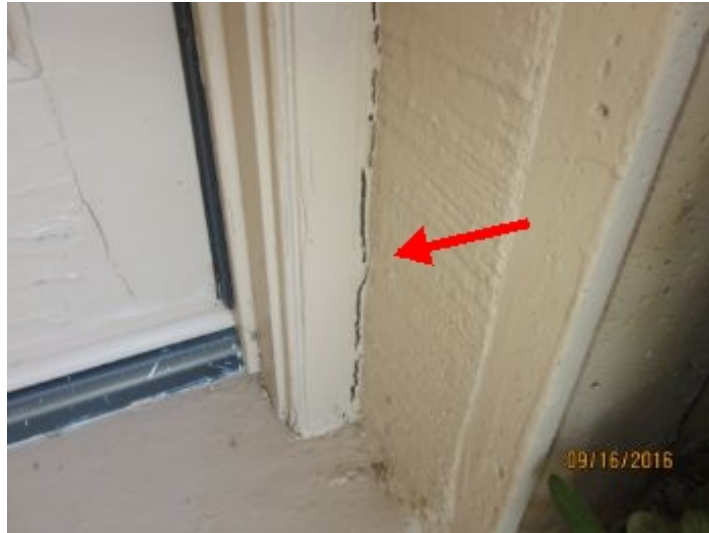
Recommend caulking around windows
