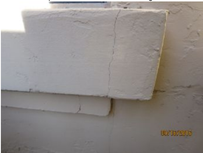
Common cracking noted
