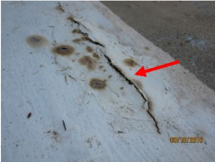
Cracking noted in foam around railings on lower roof
