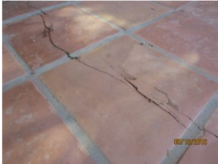
Cracked tile(s) noted on patio
