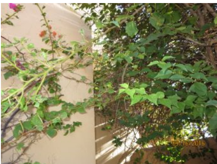
Suggest trimming vegetation away from structure.
