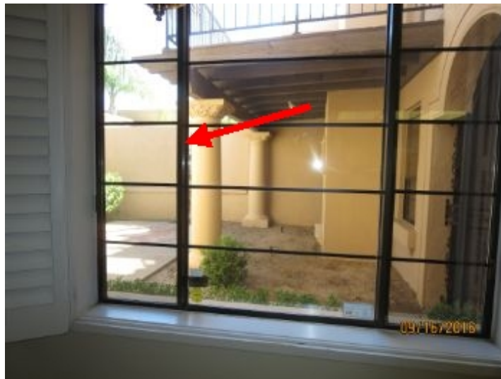
North kitchen window did not lock at the time of inspection.
