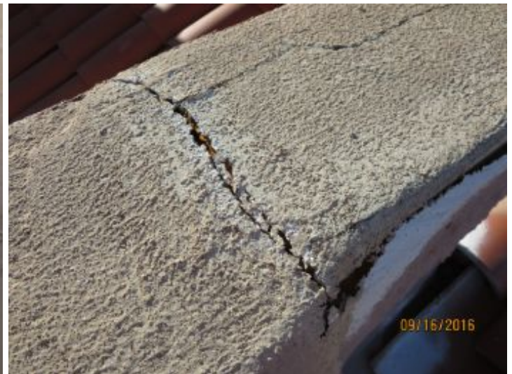
Parapet wall at perimeter of roof has several locations that need patching/caulking to prevent unwanted moisture from entering structure.
