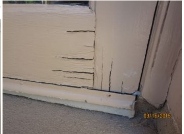
Water damage noted at base of exterior doors in both bedrooms.
