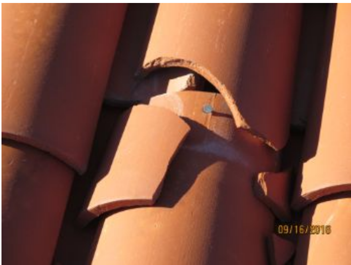
Broken tiles noted
