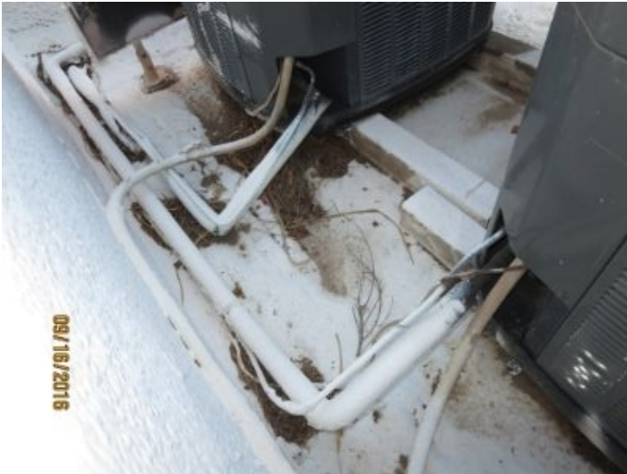
Deteriorated/missing insulation in areas. Recommend replacing the pipe wrap insulation to enhance efficiency of A/C system
