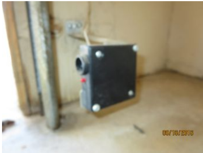
Electric eye reversed the door properly on garage opener unit at time of inspection.
