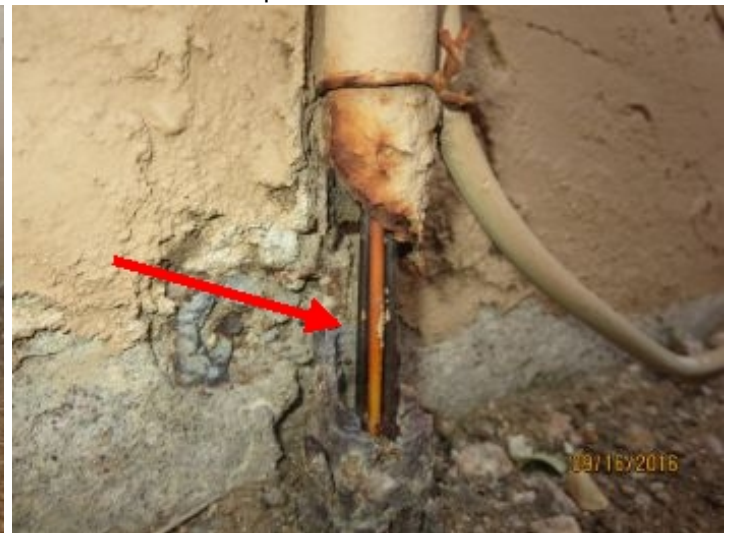
Exterior conduit is deteriorated - exposed wires noted. Recommend further review/repair by a qualified electrician.
