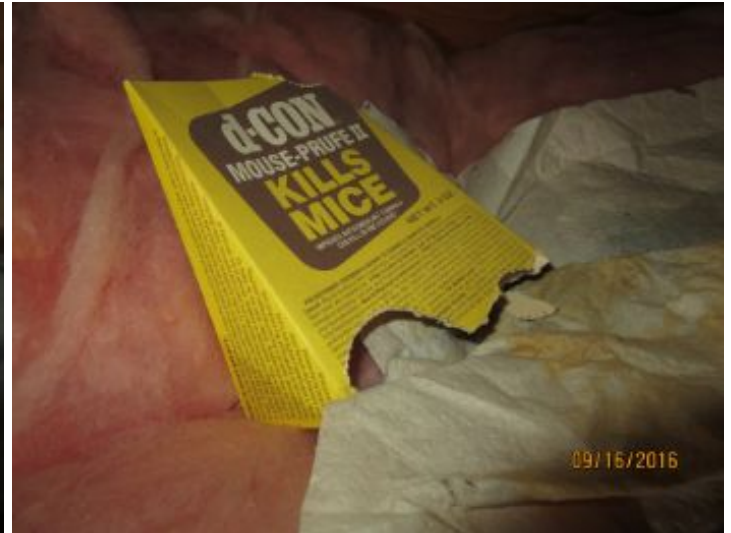
Mouse traps noted in attic. (No evidence of mice noted at the time of inspection)
