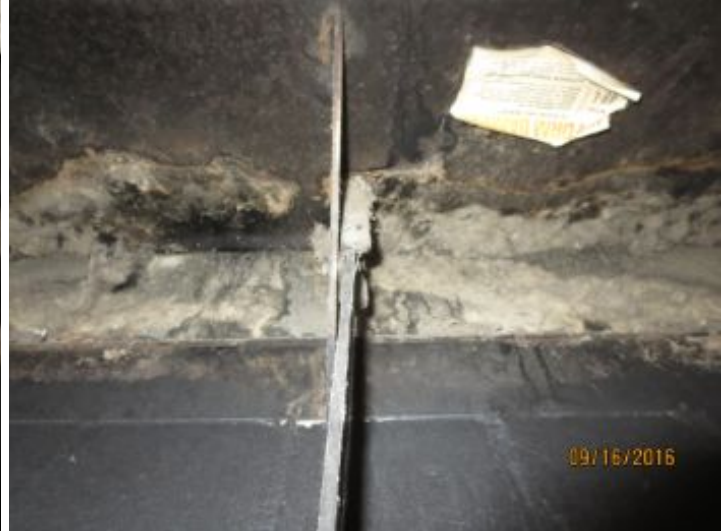
Damper was operational at time of inspection.
