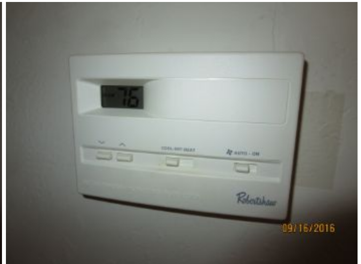
Both thermostats were functional at time of inspection
