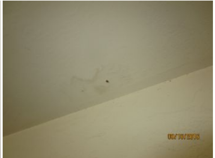
Water damage noted at garage ceiling, did not verify if leak is active or has been repaired, review and repairs are recommended by a qualified roofing contractor.
