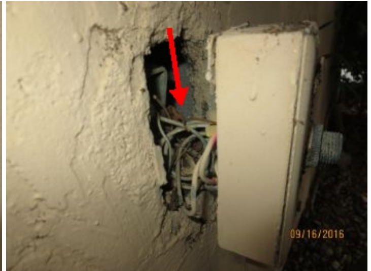
Photo cell junction box is detached from house - exposed wires noted. Recommend further review/repair by a qualified electrician
