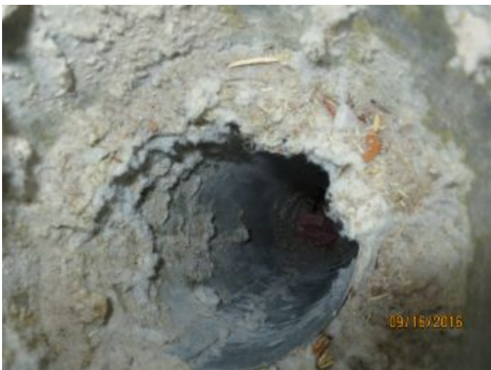
Lint buildup noted at vent cap of dryer vent termination. Suggest routine cleaning of dryer vent to prevent potential fire hazard and to enhance safety of occupants
