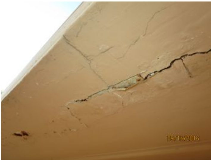
Evidence of deteriorated paint noted, recommend proper prep and painting of all exterior wood materials to extend the useful lifespan and maintain a weather tight structure.
