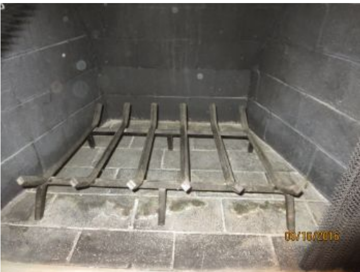
Appeared operational at the time of inspection.
