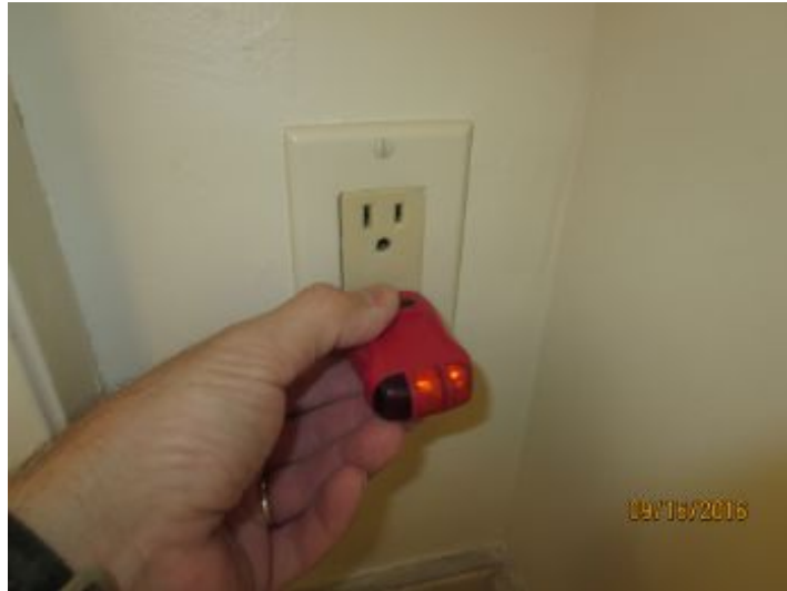
GFCI recommended in all potential wet locations
