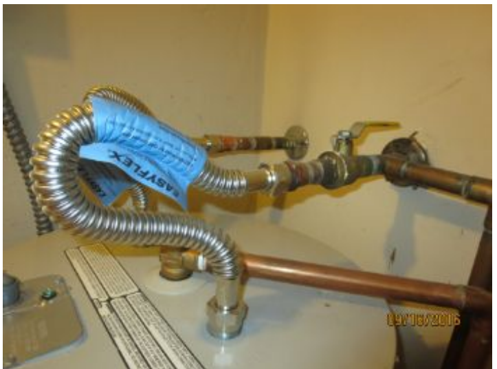
Plumbing connections were in good condition at time of inspection. No evidence of rust or corrosion.
