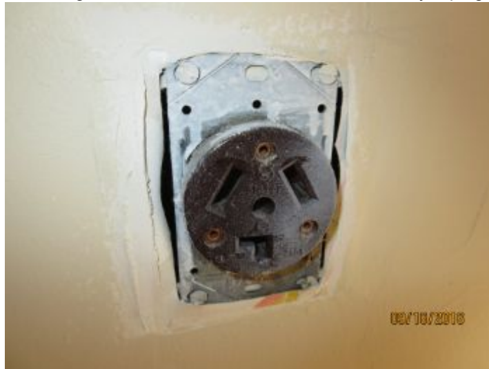
Missing 220V outlet cover in laundry room
