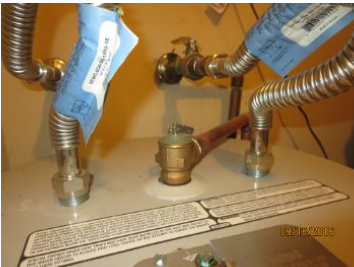
Plumbing connections were in good condition at time of inspection. No evidence of rust or corrosion.
