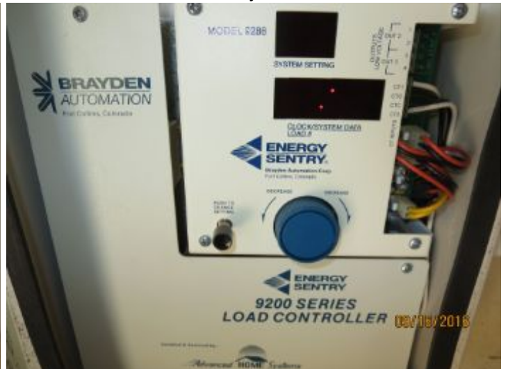
"Load Control Center" installed on interior garage wall. Not part of home inspection - recommend further review by a qualified electrician.
