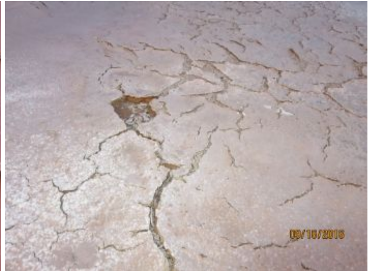
Alligatoring or cracking of roof surface noted in one or more location(s)
