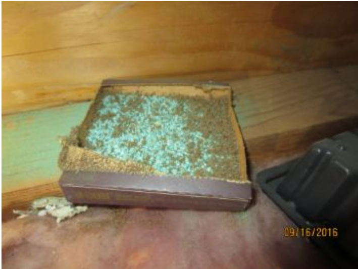
Mouse traps noted in attic. (No evidence of mice noted at the time of inspection)
