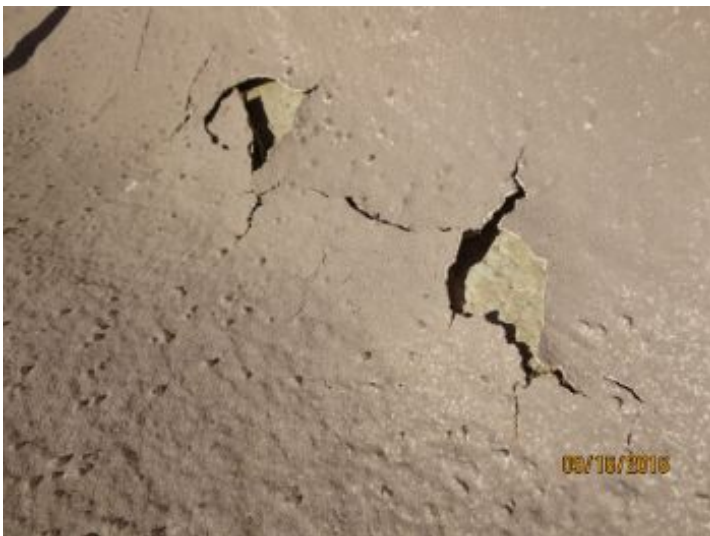
Holes/deterioration noted in foam in one or more location(s) Recommend further review/repair by a qualified roofing contractor.
