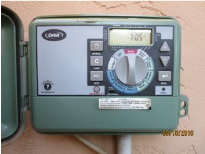
Timer location: East exterior side of house
