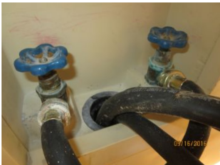
The hot and cold supply shutoff valves for the washing machine appear to be in good condition with little or no corrosion/rust present at time of inspection
