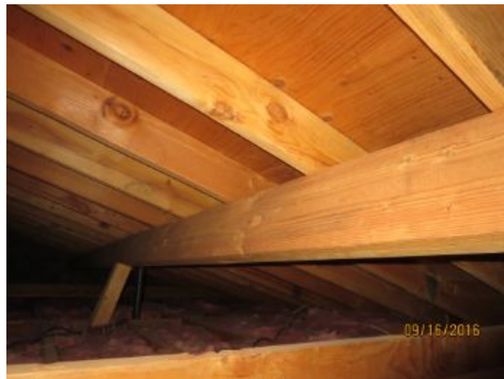
Roof structure appeared to be in good condition with no visible evidence of water stains or structural issues in the areas that I had access to.
