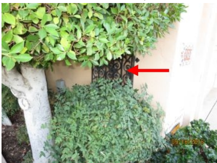
Recommend trimming shrubs and tree to allow easier access to electric panel.
