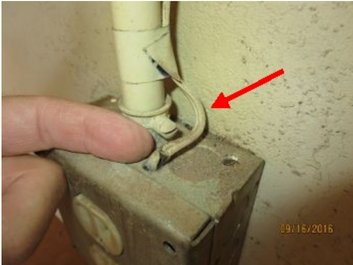
Improper wiring practices observed at one or more locations. Recommend review and repair of spliced and taped wires by a Qualified Electrician.
