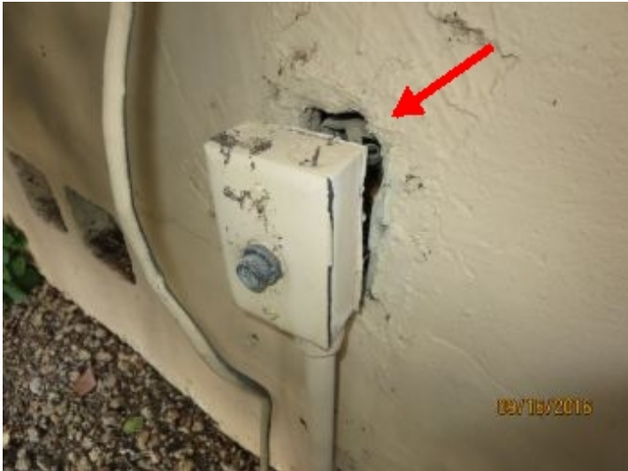
Photo cell junction box is detached from house - exposed wires noted. Recommend further review/repair by a qualified electrician
