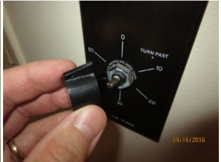
Whirlpool timer knob was stripped at the time of inspection.
