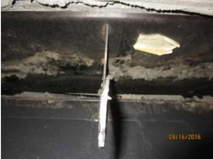
Damper was operational at time of inspection.
