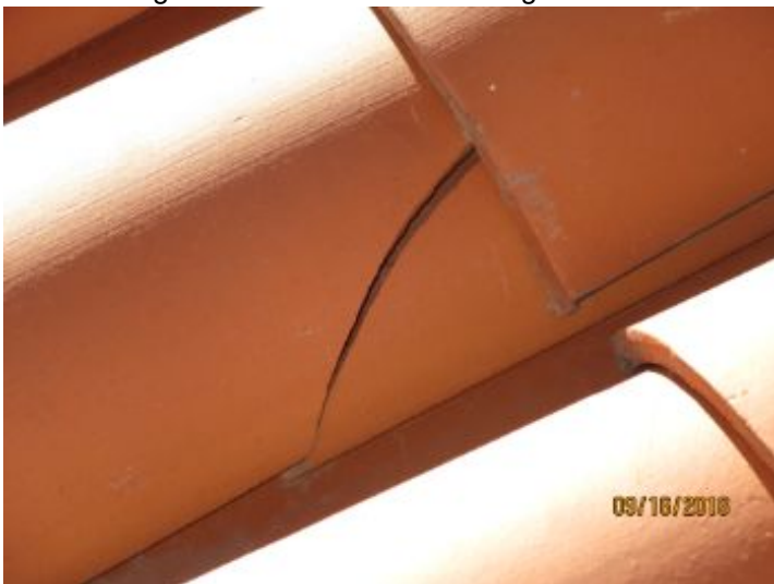
Cracked tiles noted
