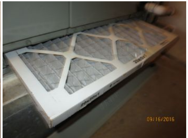
Furnace filter location: Furnace base. Size: 20" x 20"
