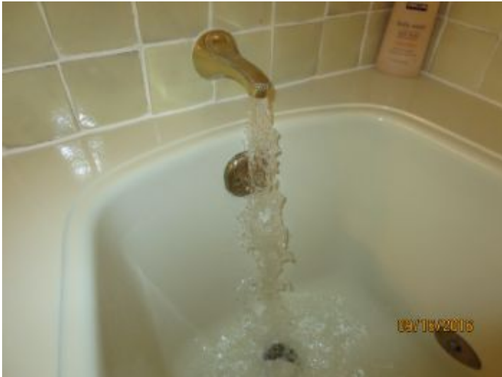
2nd floor guest bathtubs were functional at time of inspection
