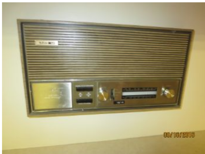
Home appears to have a intercom and/or audio system installed.
