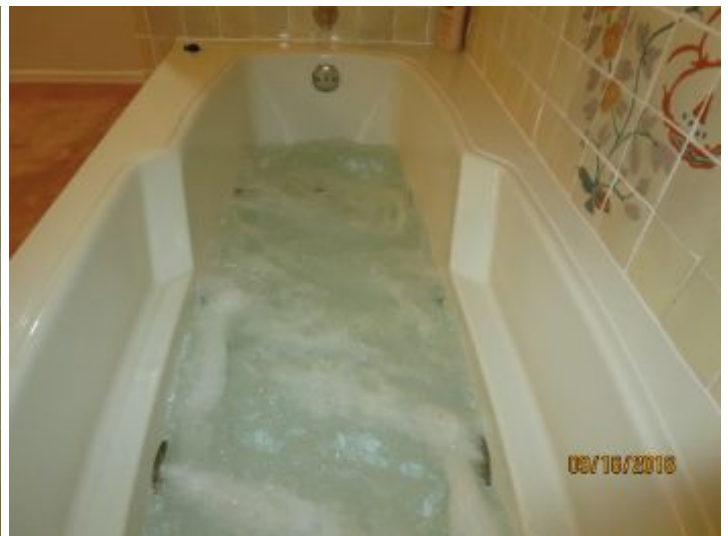
Whirlpool tub operated at time of inspection
