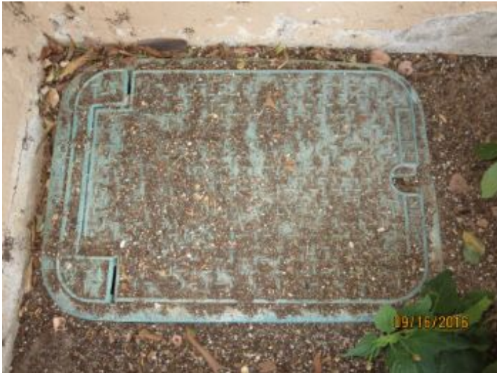
Valve box 1 location: East side of garage
