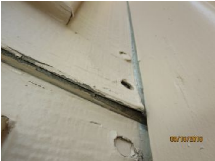
Damaged/deteriorated exterior garage door panels noted.
