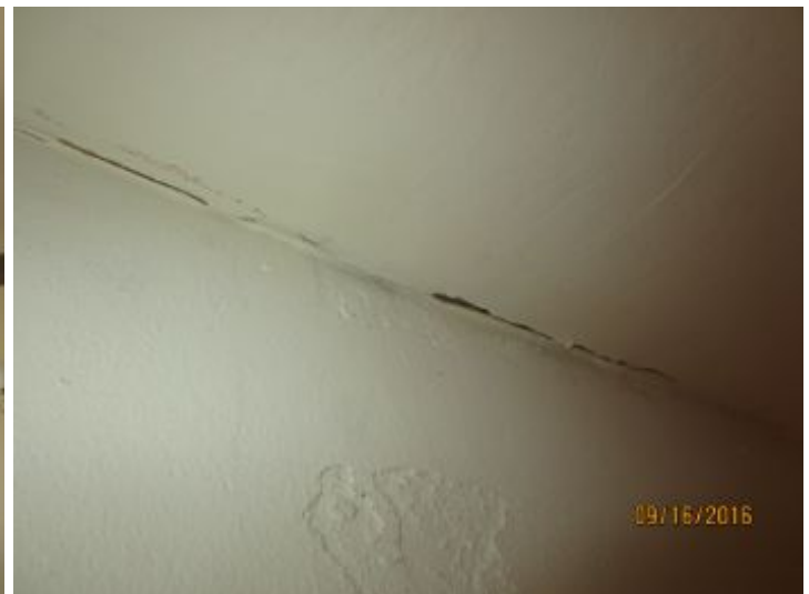
Evidence of past leaking at ceiling above fireplace in northeast bedroom.,did not confirm that leak has been properly repaired. Recommend monitor area after heavy rain and repair as needed by qualified roofing contractors.
