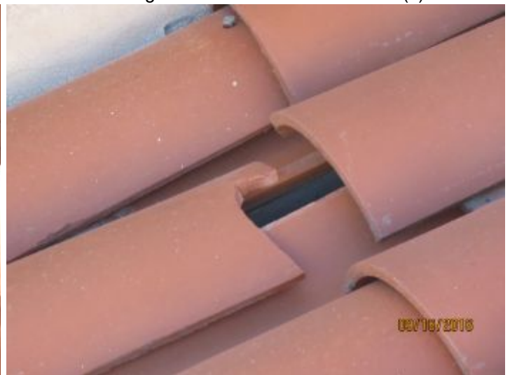
Broken tiles noted
