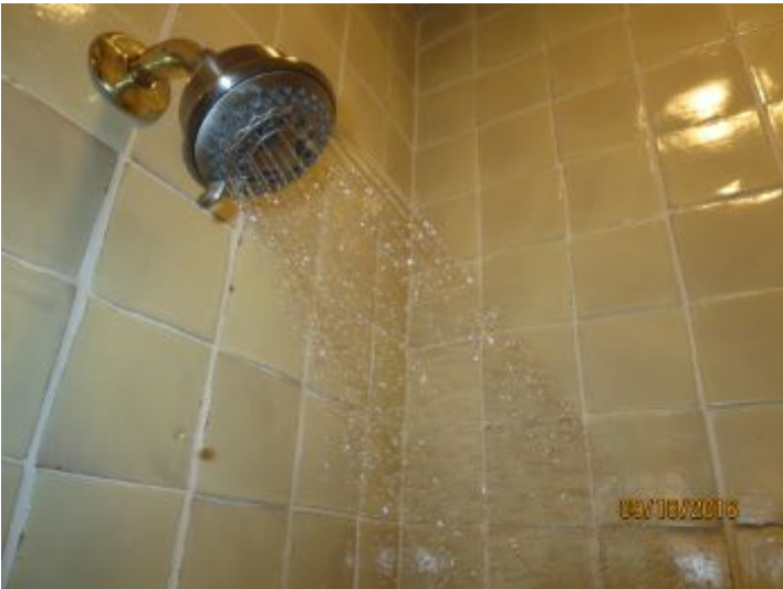
The 2nd floor guest showers were functional at time of inspection
