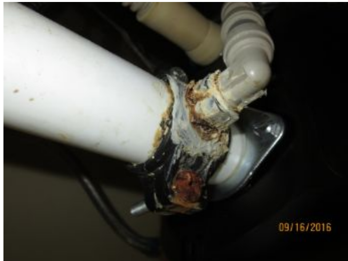
Heavy rust noted at plumbing connection under kitchen sink.
