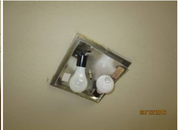
Missing light globe in garage
