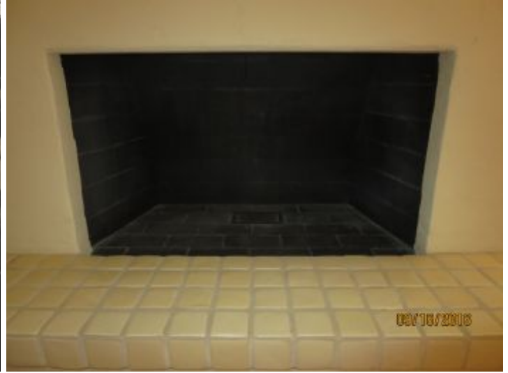
Fireplace appeared functional at the time of inspection.
