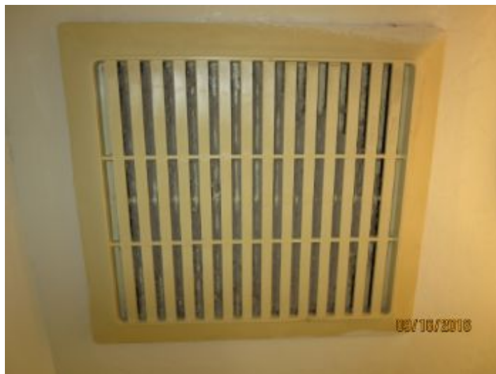
Dirty - needs vacuuming
