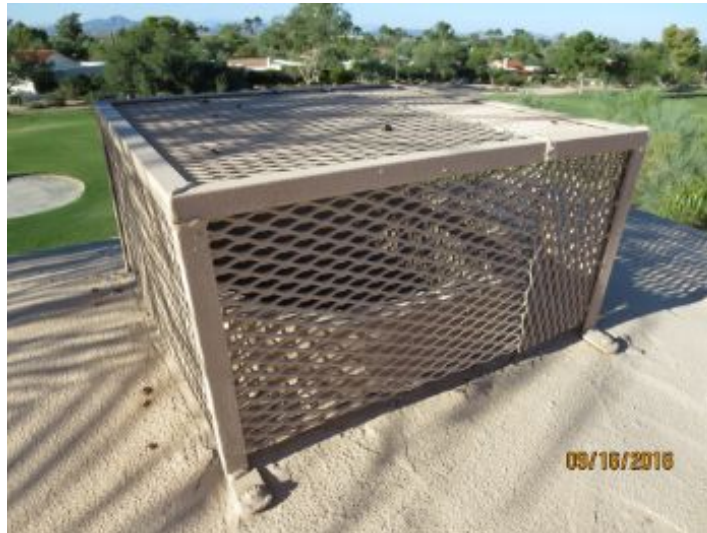
Spark arrestor/rain caps were present at the time of inspection
