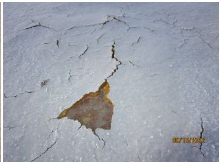
Holes/deterioration noted in foam in one or more location(s) Recommend further review/repair by a qualified roofing contractor.
