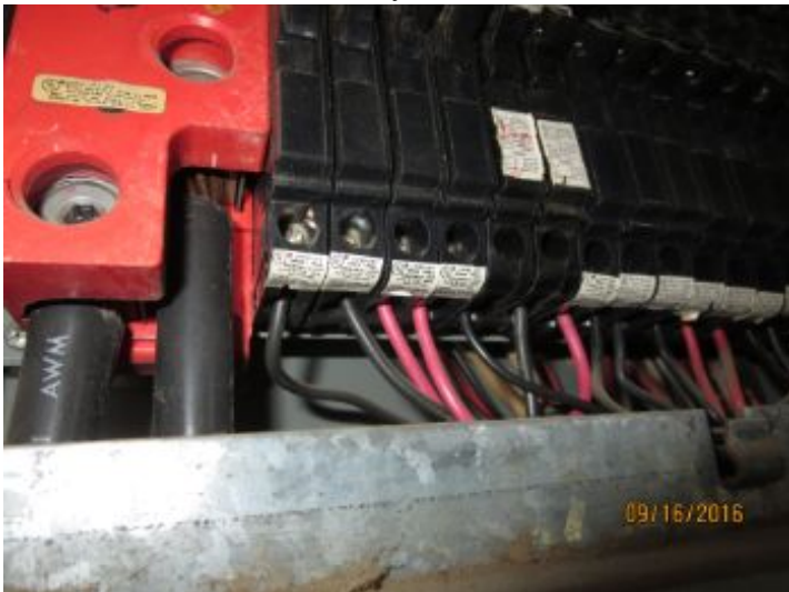
The branch wires visible in the panel are copper and are in satisfactory condition.
