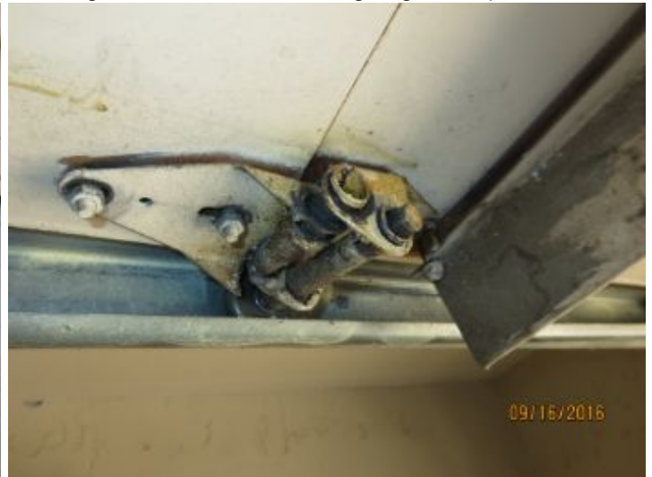
Damaged/bent garage roller noted.
