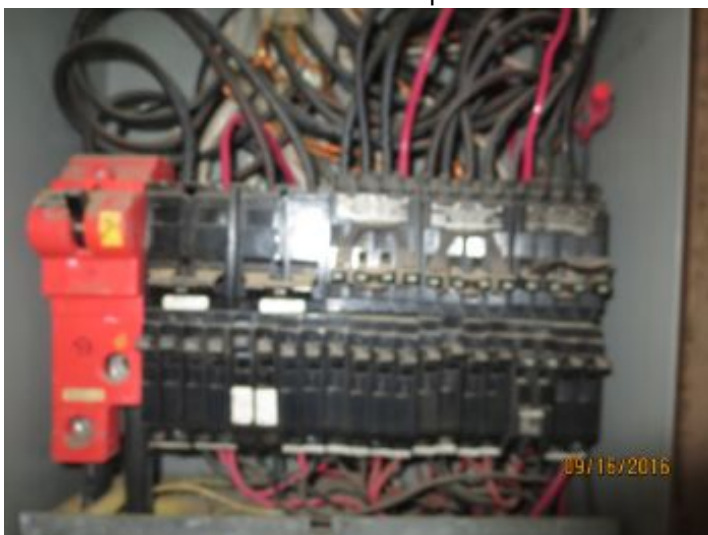
The branch wires visible in the panel are copper and are in satisfactory condition.
