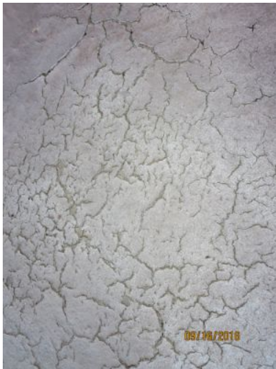
Alligatoring or cracking of roof surface noted in one or more location(s)
