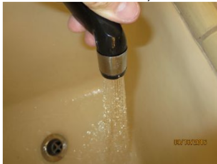
The utility sink spray wand did not operate at the time of inspection.
