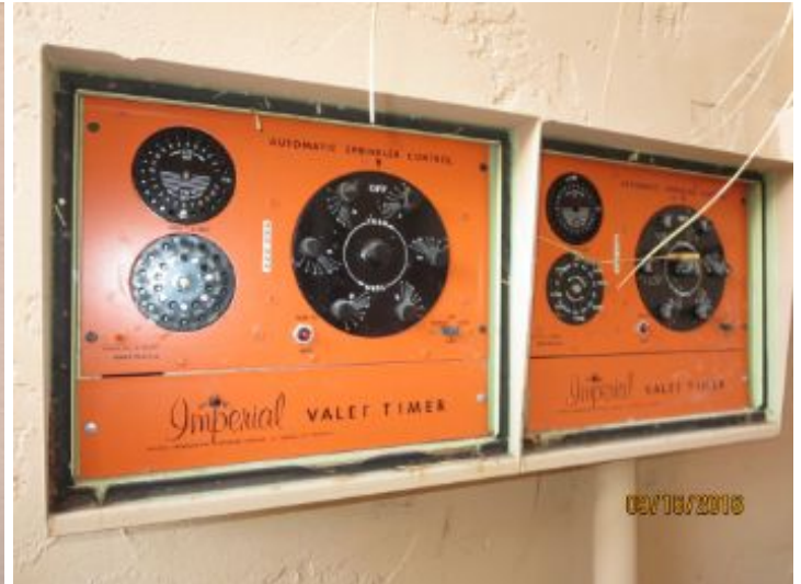
Timer location: East exterior side of house
