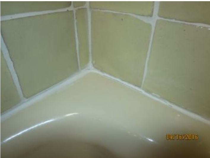
Recommend grout in one or more location(s)
