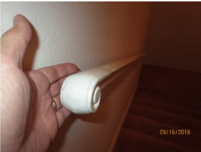
Current building standards require that the handrail returns to the wall to prevent loose clothing or a purse strap (for example) from getting caught and potentially presenting a safety hazard. This may not have been the standard when this home was built. Recommend upgrading handrail to enhance safety of occupants.
