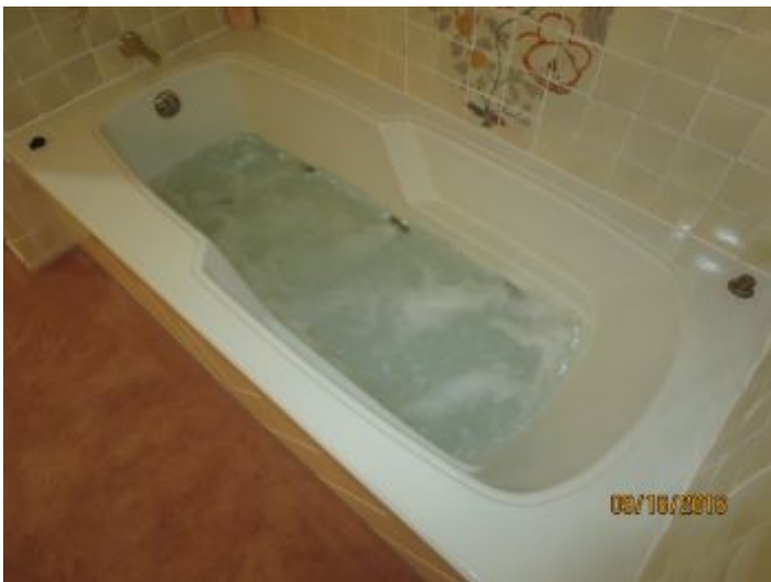
Whirlpool tub operated at time of inspection
