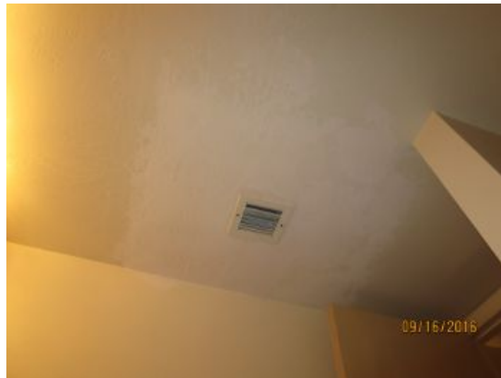
Patched areas noted
