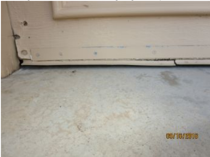
Garage door bottom weather stripping is deteriorated.
