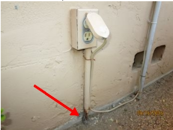
Exterior conduit is deteriorated - exposed wires noted. Recommend further review/repair by a qualified electrician.
