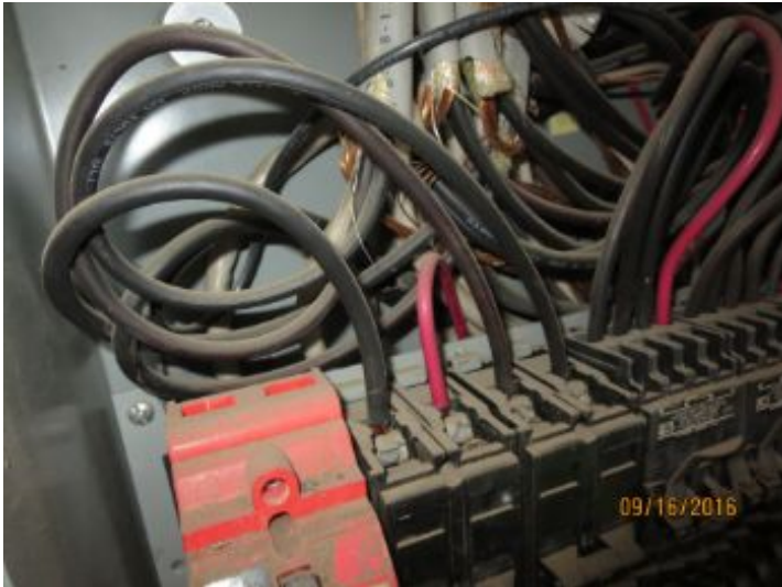
The branch wires visible in the panel are copper and are in satisfactory condition.
