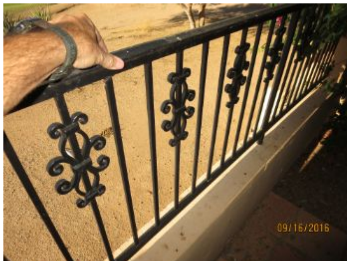
Loose railing noted at back balcony.
