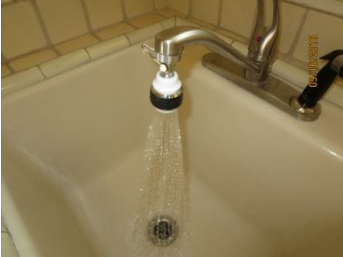
Laundry room sink faucet was loose at sink connection.
