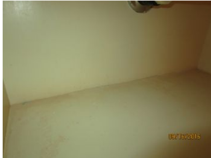
Evidence of past leaking on bottom of cabinet
