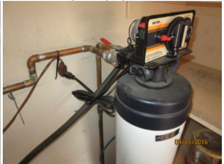
Water softener and/or filtration system present in garage.
